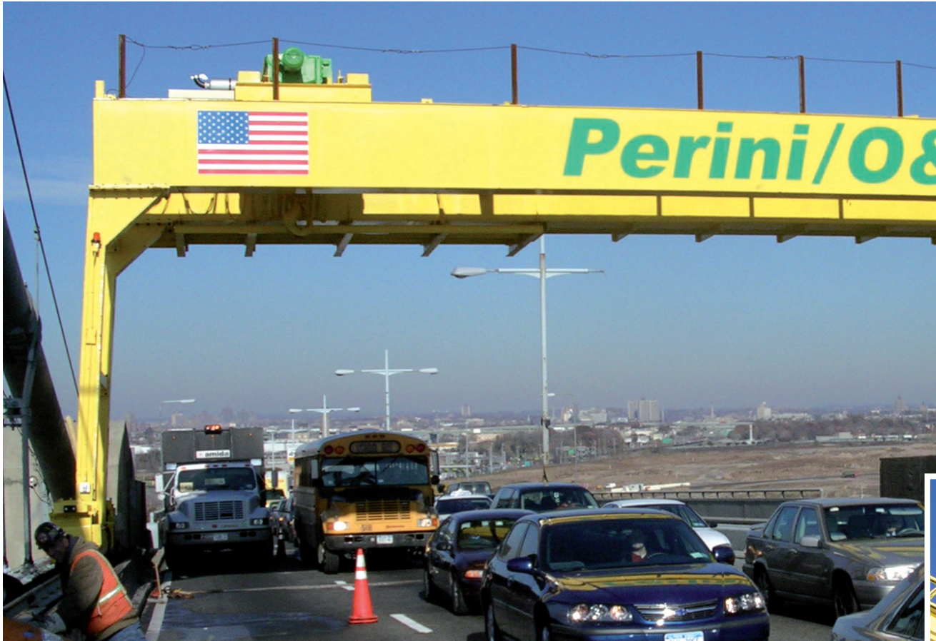
Perini Corporation and O&G Industries teamed-up with North American Industries, Inc. (NAI) to design and manufacture four gantry cranes
